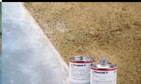
6 Construction joints should be closed by adhesion using a reactive resin system (e.g. Thixopont, F) prior to laying the floor covering
